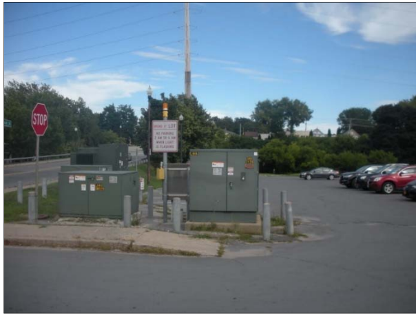
Photo #7-1 (facing east): View of BSMPL with the Saranac River and the Broad Street Bridge in the background.
